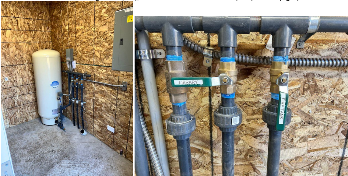
Pressure tank set up (left) and valve shut off (right).
